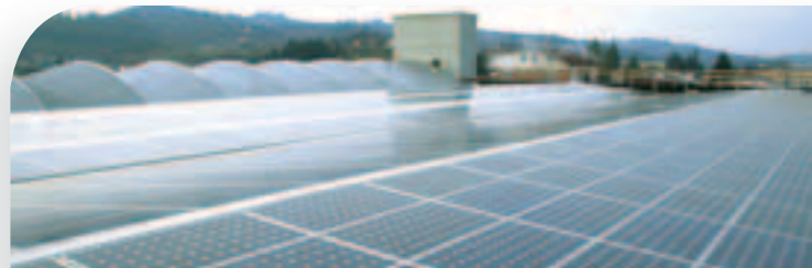
200 kWp Piemonte (AT)
